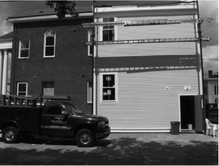
Rear of building exterior - addition is for new second stair and exit. It is finished with cement plank siding.
