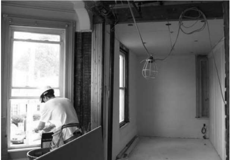
Second floor - existing window openings are retained and windows replaced. Walls and ceilings in this room are new. Room will be a common lounge.
